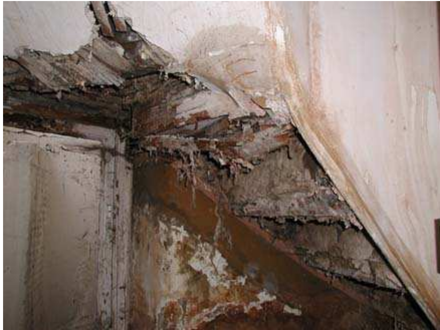
Extensive timber decay caused by dry rot (Serpula lacrymans)
