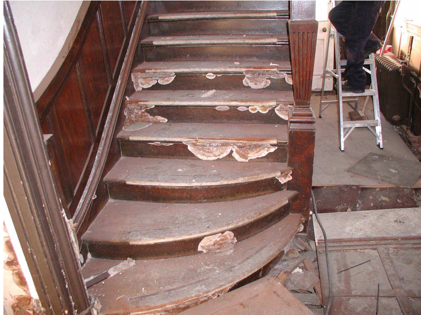
Dry rot fruiting bodies to timber staircase, causing extensive structural damage.
