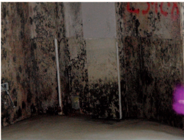
Fig. 1. Toxic mould on Gyproc plasterboard.
