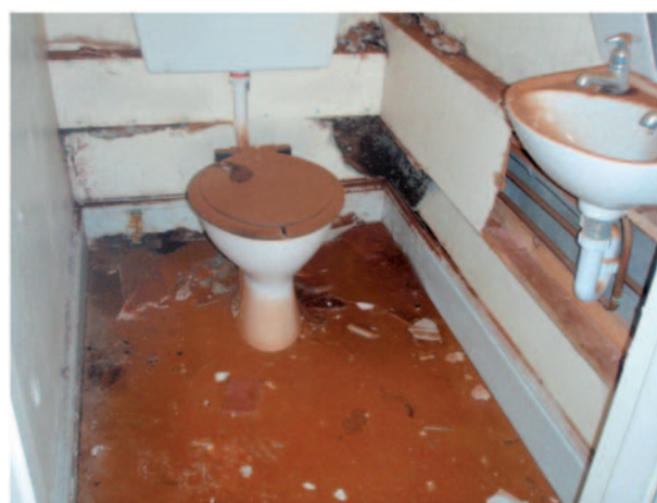
Fig. 3. Dry rot spores covering the surfaces.
